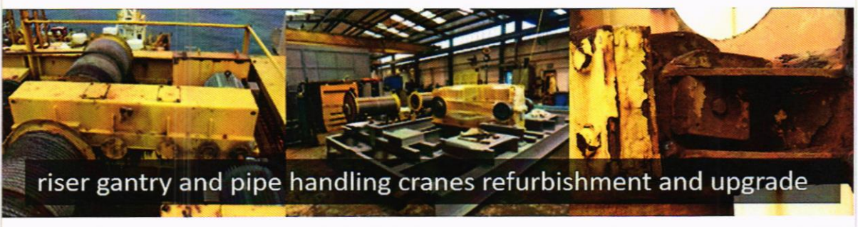
Surface BOP and handling system
